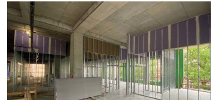
This open and airy space is the future reception area for the college's administrative offices.
