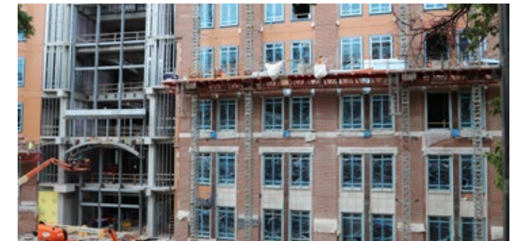
Workers add the elegant brick exterior to the north side of the new building. This area will be home to first-year studies and the college administration.
